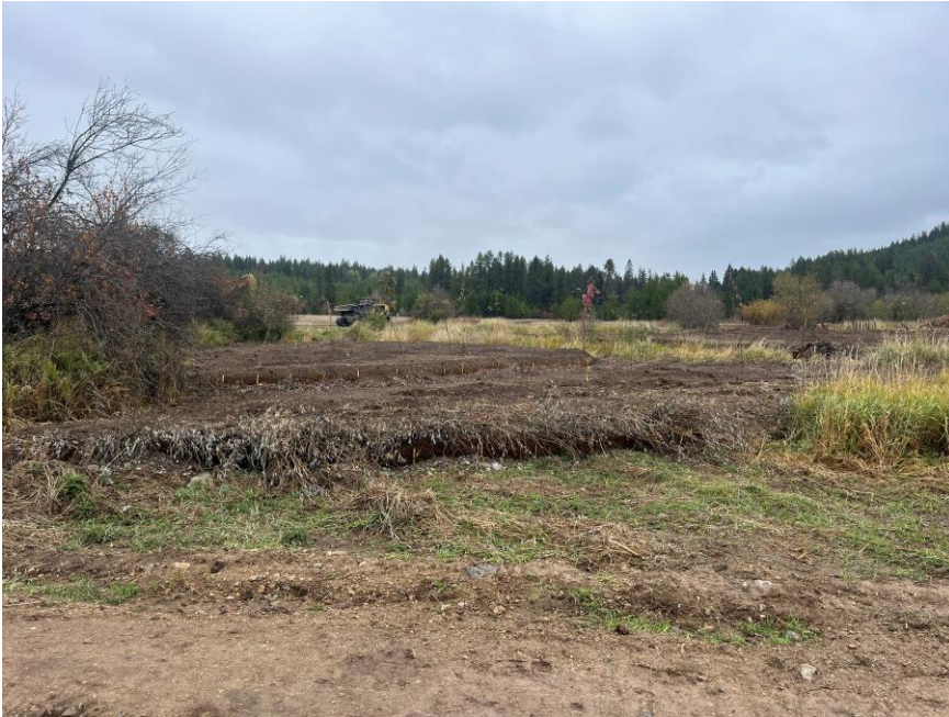
Photo 6. Soil salvaged from floodplain grading was mixed with imported gravel to construct soil encapsulated lifts to create new streambanks and floodplain surfaces. Note live willow cuttings were placed between lifts to increase roughness and provide root mass for promoting long-term stabilization of the new streambanks.
