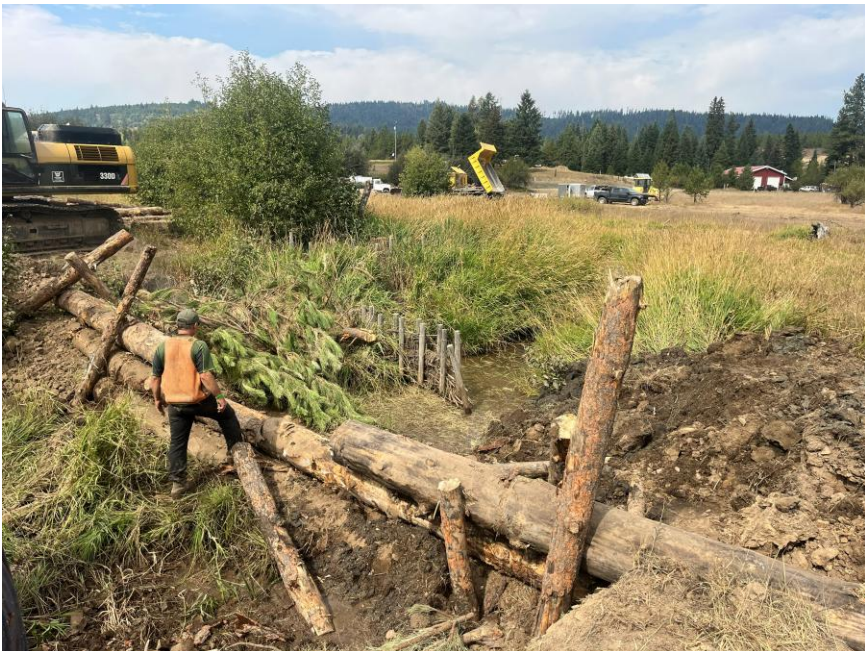
Photo 7. Construction of an instream structure designed to emulate the flow obstruction effects of natural wood jams and beaver dams. At each location, the active stream channel was plugged with large wood buried in the stream bed and banks and covered with imported stream gravels. Channel was fully dewatered during construction.
