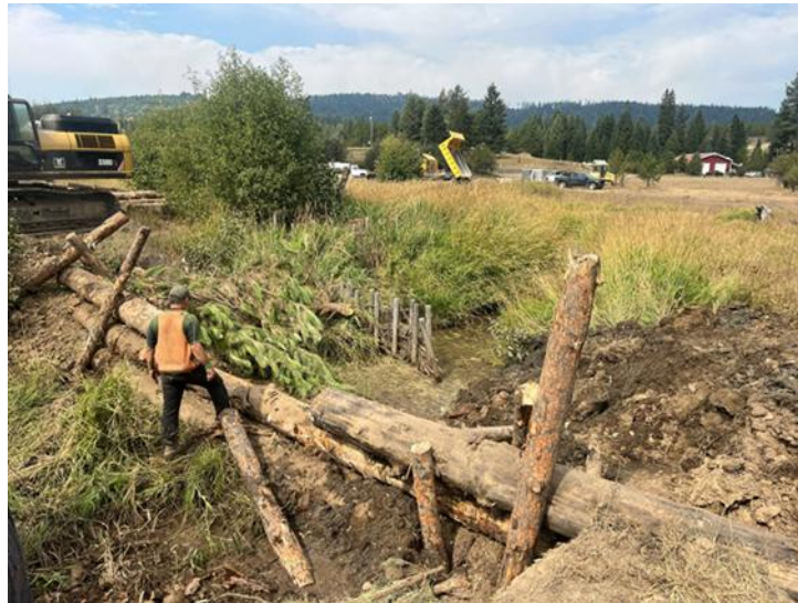
Construction of an instream structure designed to emulate the flow obstruction effects of natural wood jams and beaver dams
