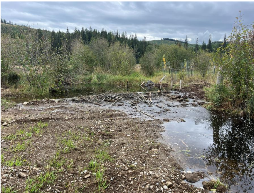
Photo 9. (Looking upstream) Beaver began building a starter dam directly on top of an instream structure shortly following completion of construction in September 2025.
