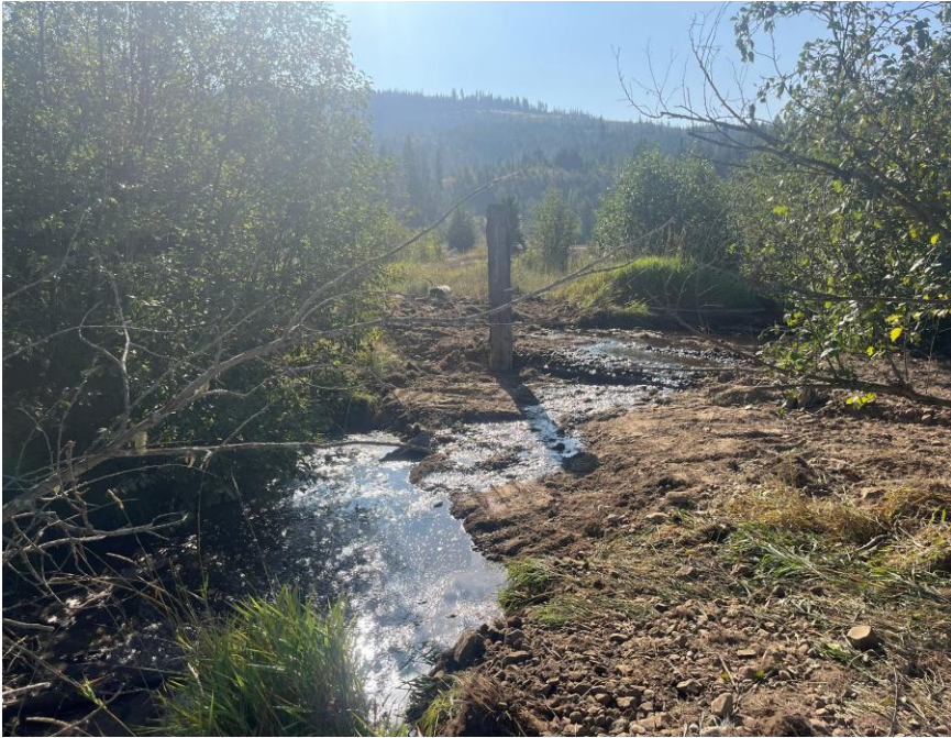
Photo 8. Completed instream structure looking upstream during baseflow condition in September 2025. Channel is fully wetted and connected to the valley bottom floodplain.
